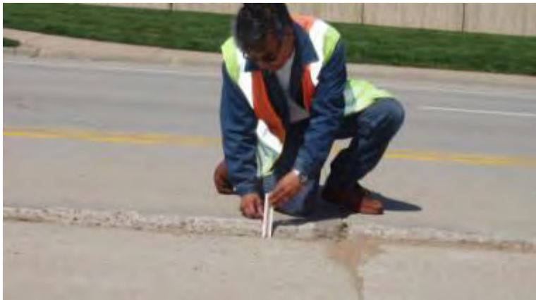
Figure 2. A faulted longitudinal joint.
