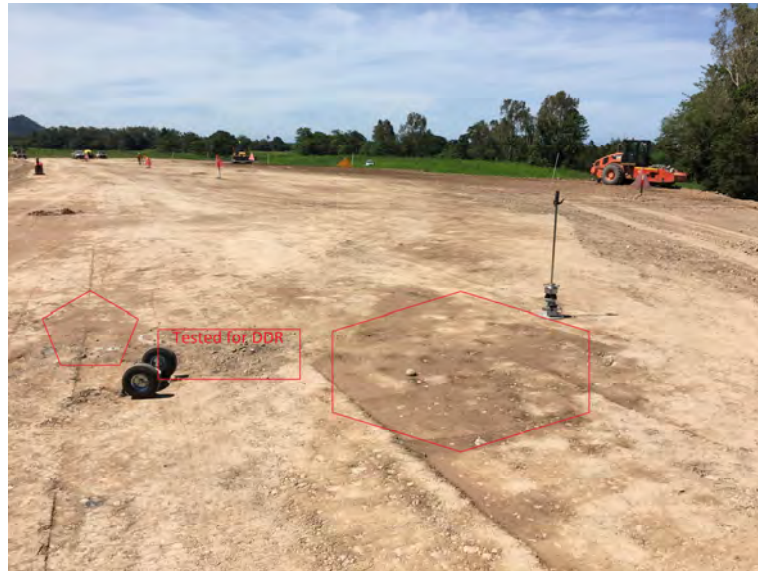
Figure 6-3 Localised wet area and Testing Area
